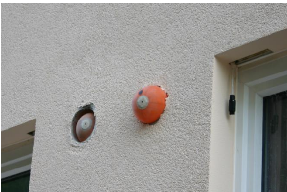
Temporary sealing of the outdoor air and exhaust air openings of the ventilation system during the measurement
